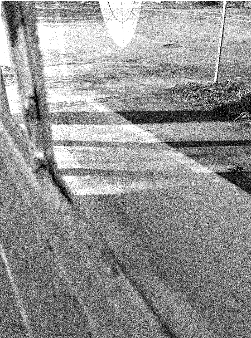
Window rot bad glazing north side
