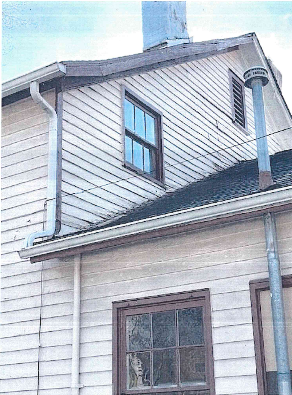
Close up of chimney deterioration and fascia rot close up.
