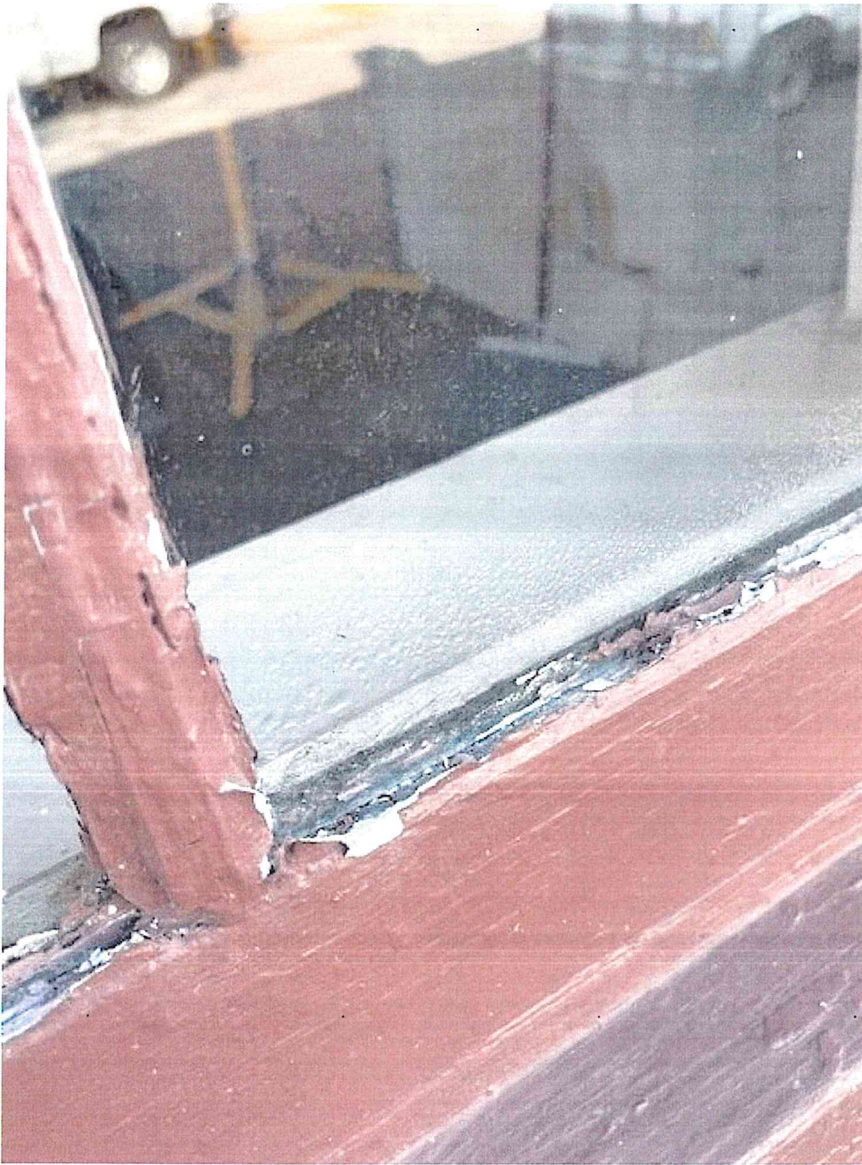
Window rot bad glazing north side
