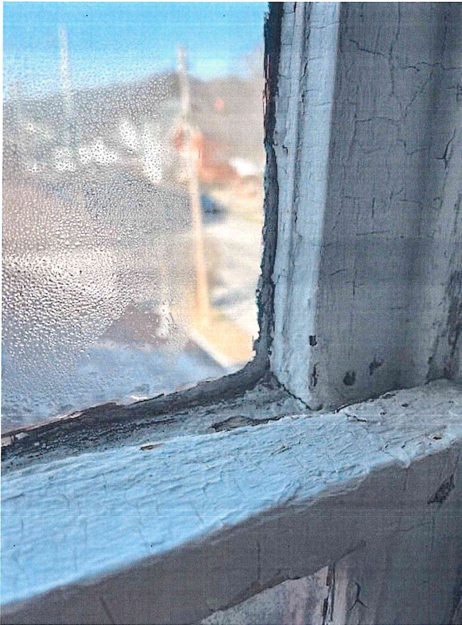
Rot in window from inside (if zoomed in you can see through the sash by the pane)
