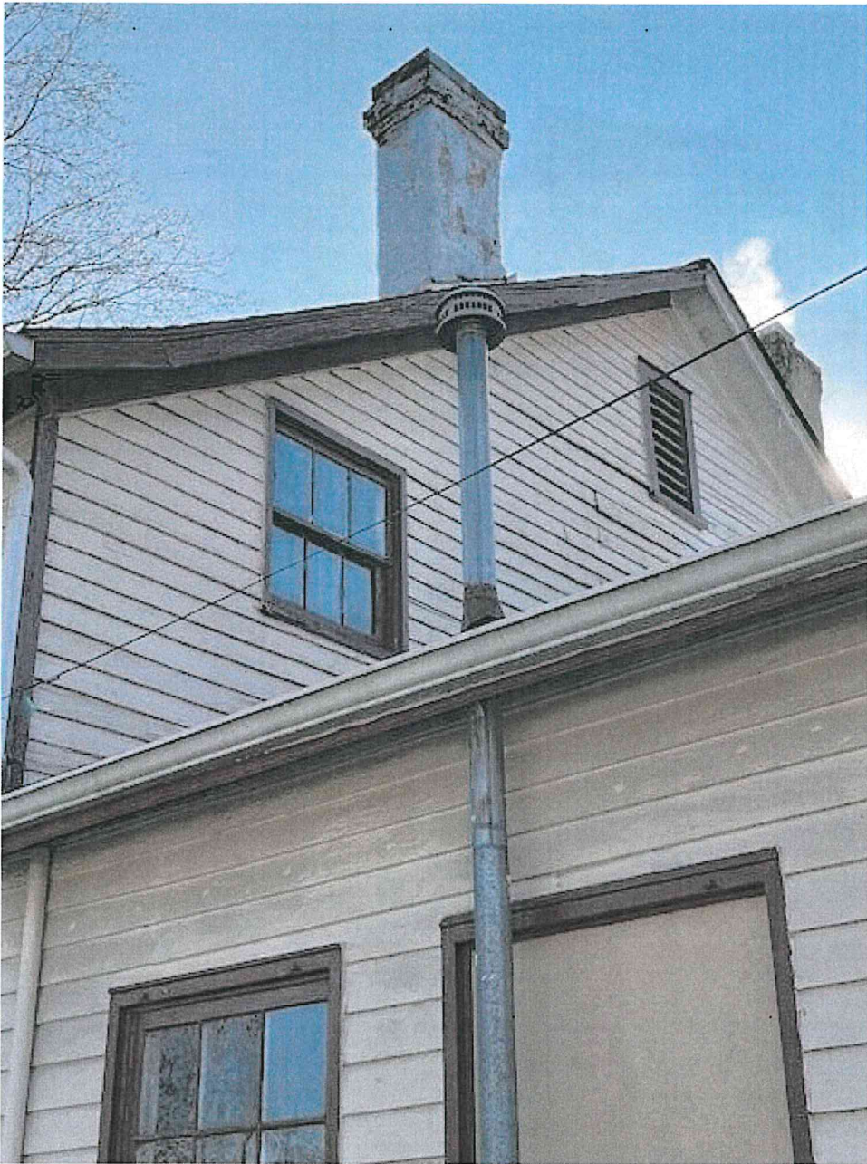
Siding / facia rot west side
