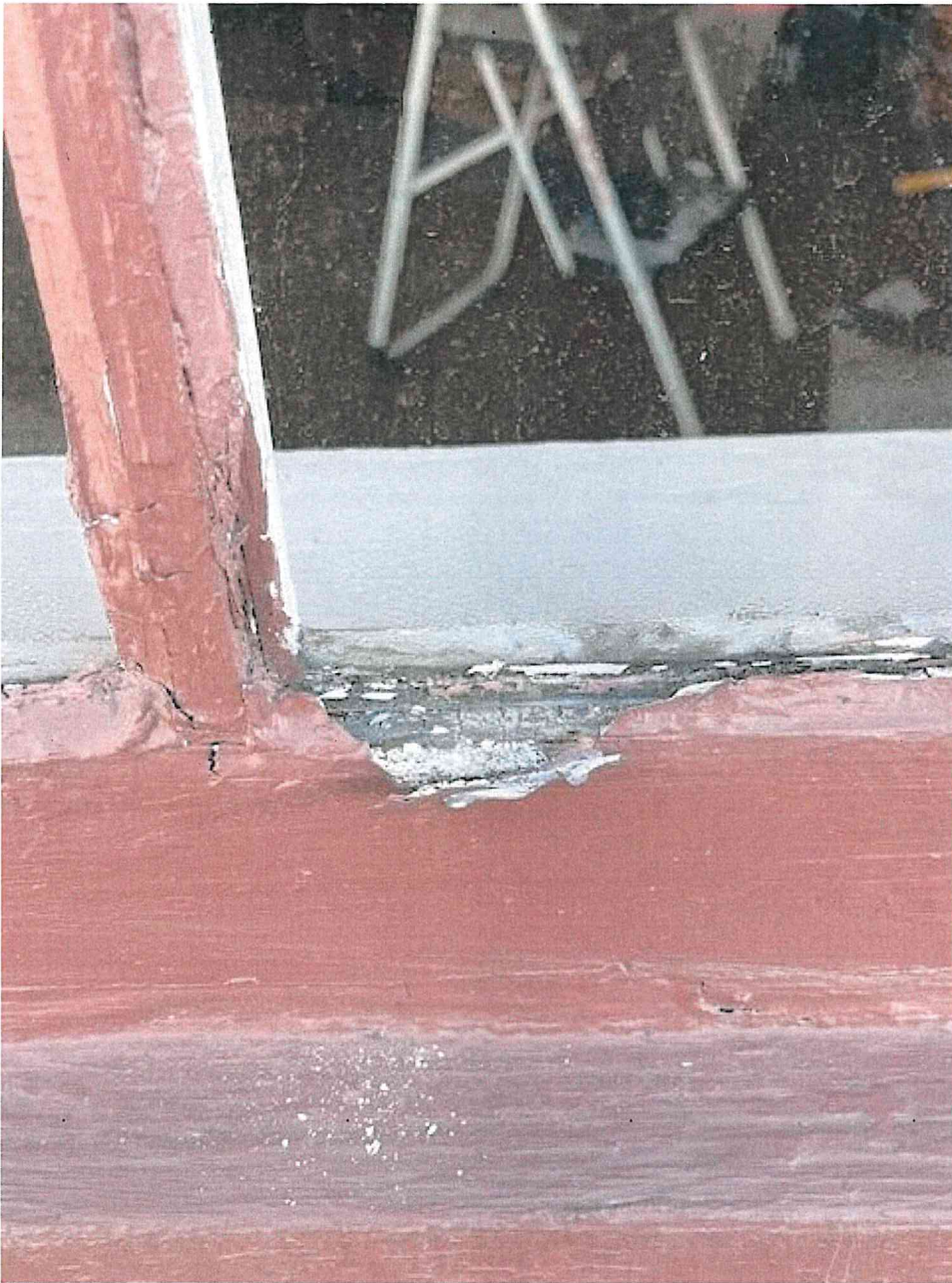
Window rot bad glazing north side
