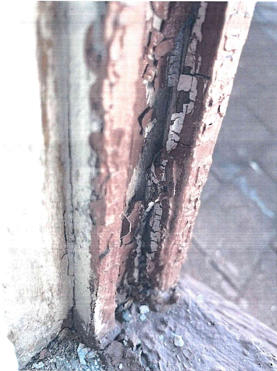
Bad glazing on window with rot
