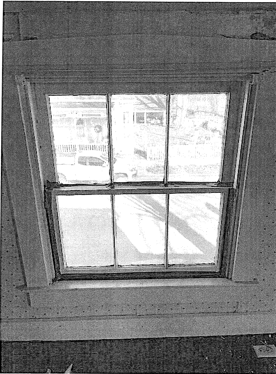
Window rot north side
