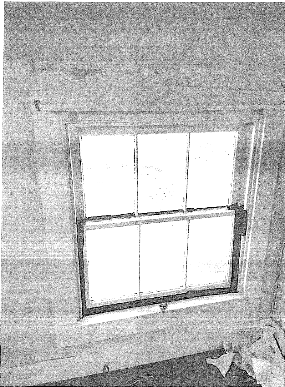
Bedroom 2 with window safety issue because of height from floor.
