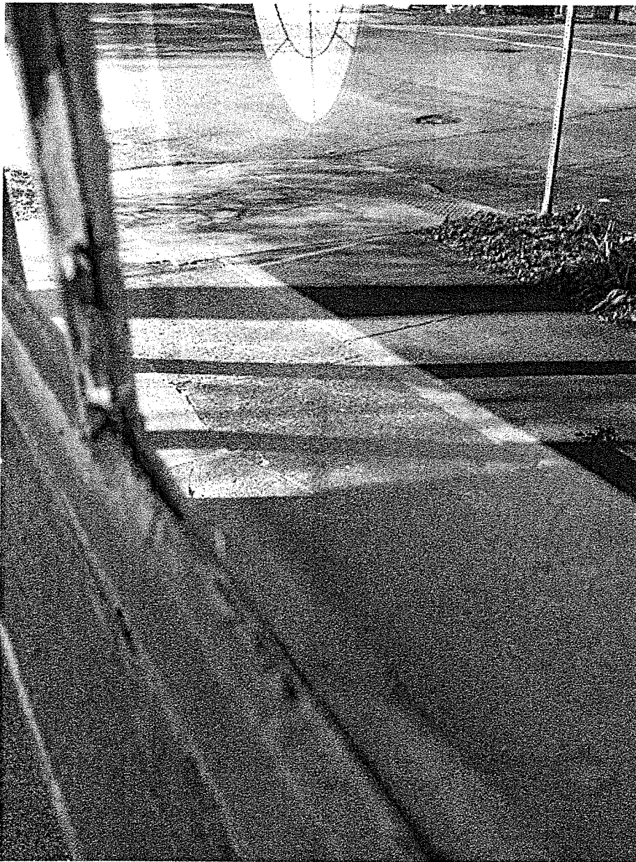
Window rot bad glazing north side
