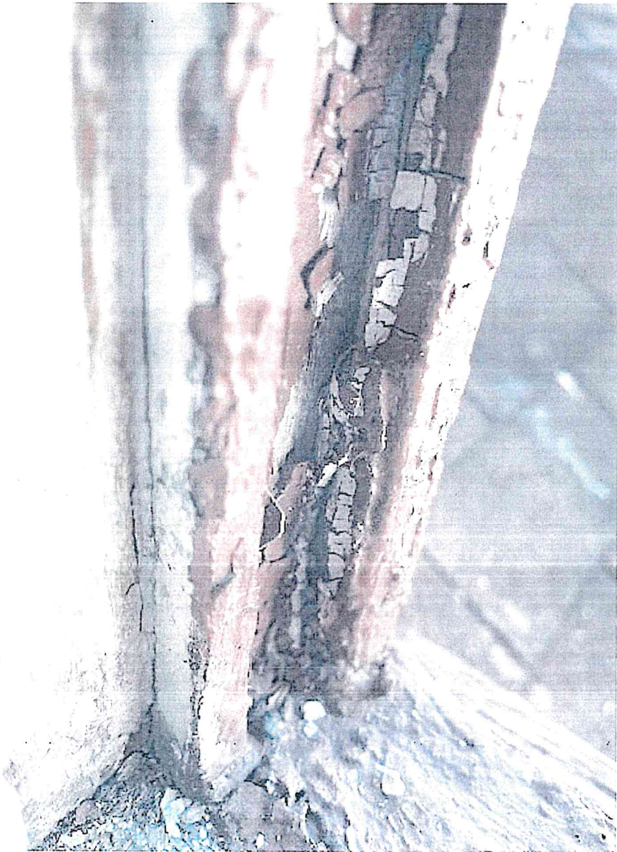
Bad glazing on window with rot
