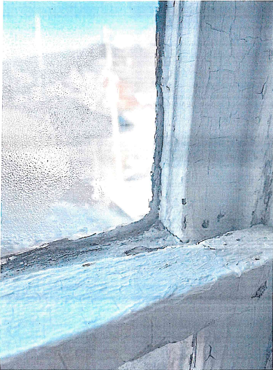
Rot in window from inside (if zoomed in you can see through the sash by the pane)
