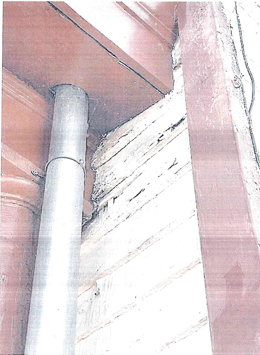
Window rot bad glazing north side
