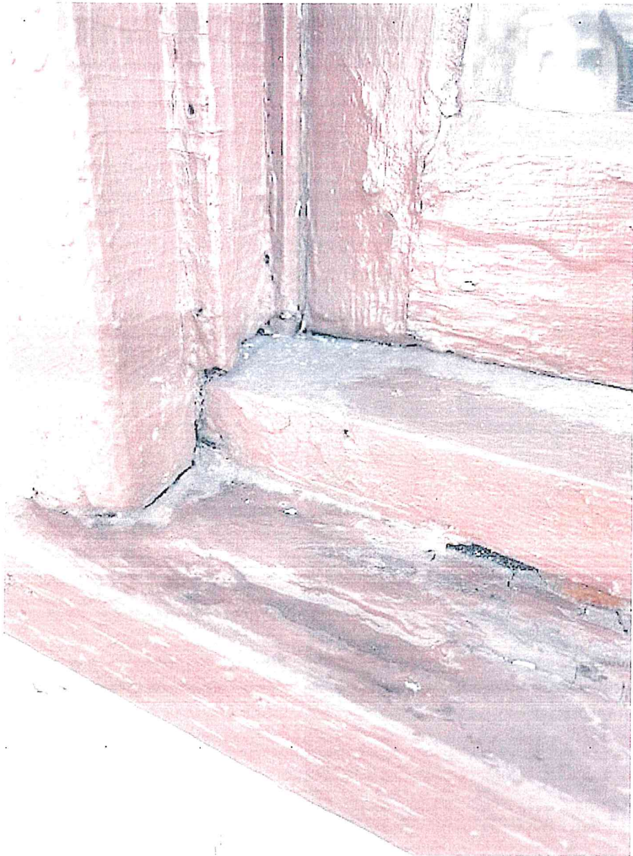
Chimney deterioration west side.
