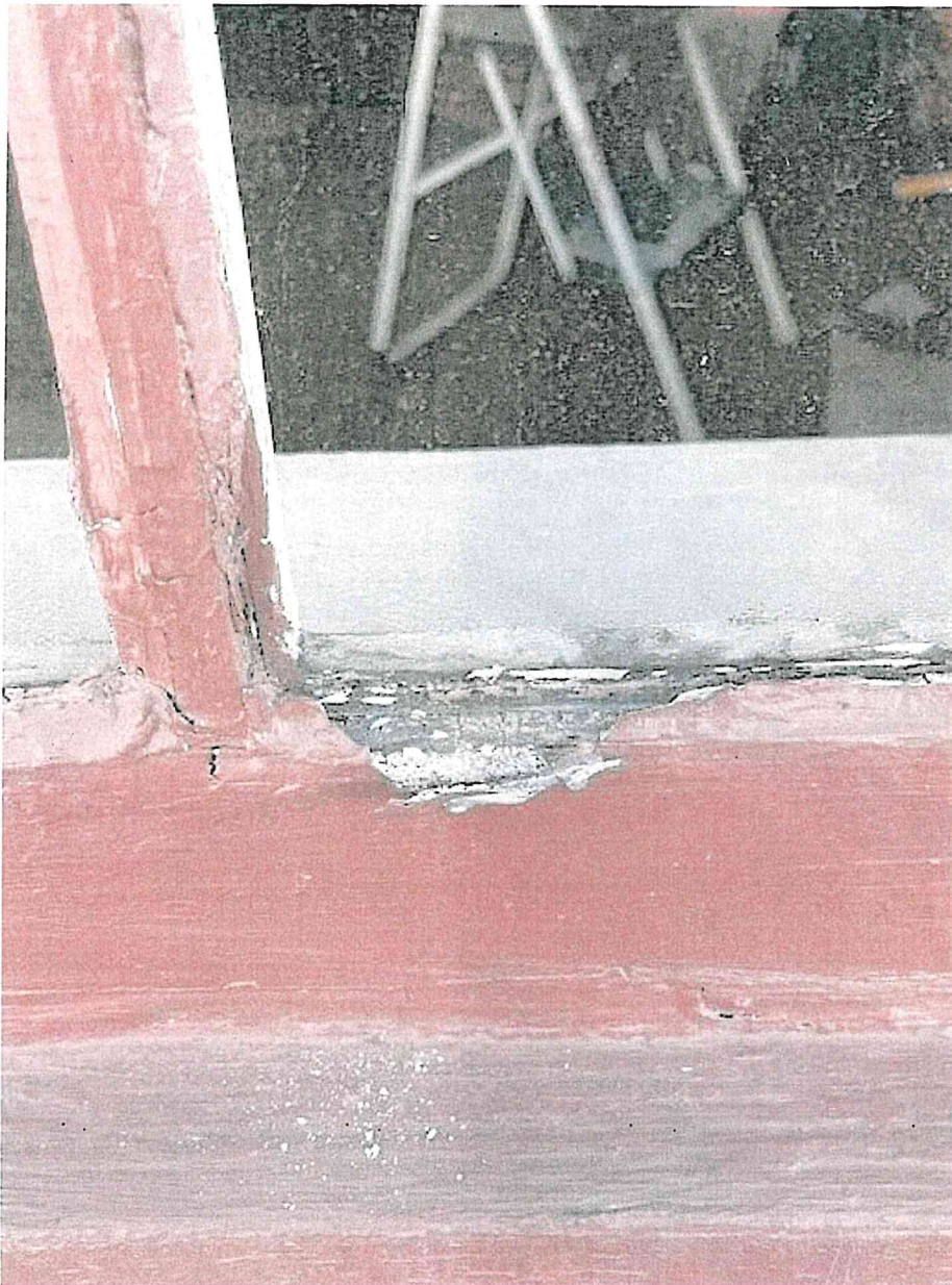
Window rot bad glazing north side
