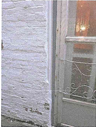
Brick altered opening 24" from bottom.
