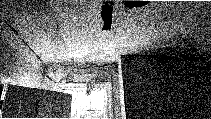
More examples of structural damage which requires removal of plaster from all walls and ceiling for further evaluation.
