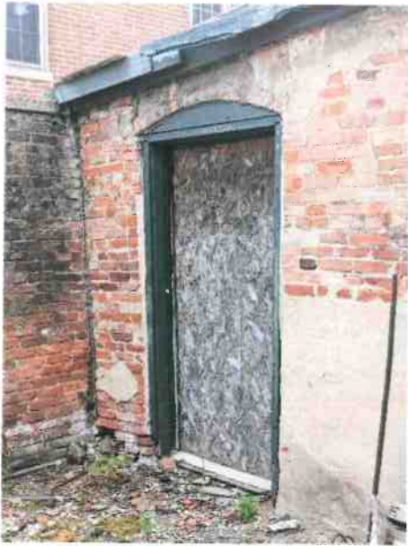
Door missing Southeast corner of Donkey Barn, more evidence of rotted fascia board
