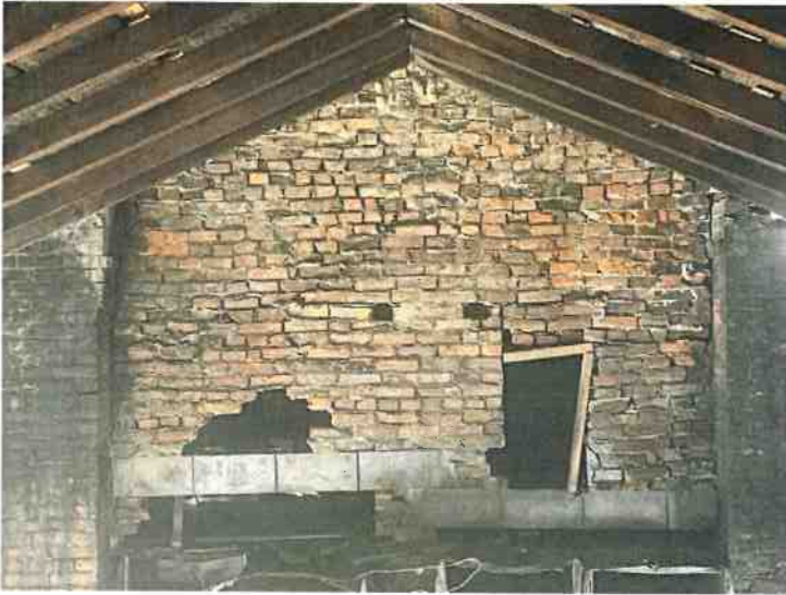
Current state of retaining wall in attic which connects to two structures is worrisome. This is where the roof line changes for the house going east.
