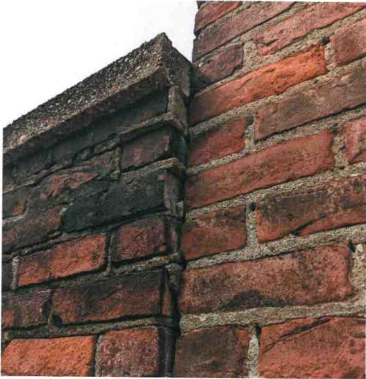
Evidence of leaning wall along alley
