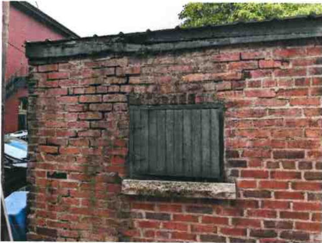
Window cover doesn't close on Donkey barn, rotted fascia board, and brick work needed
