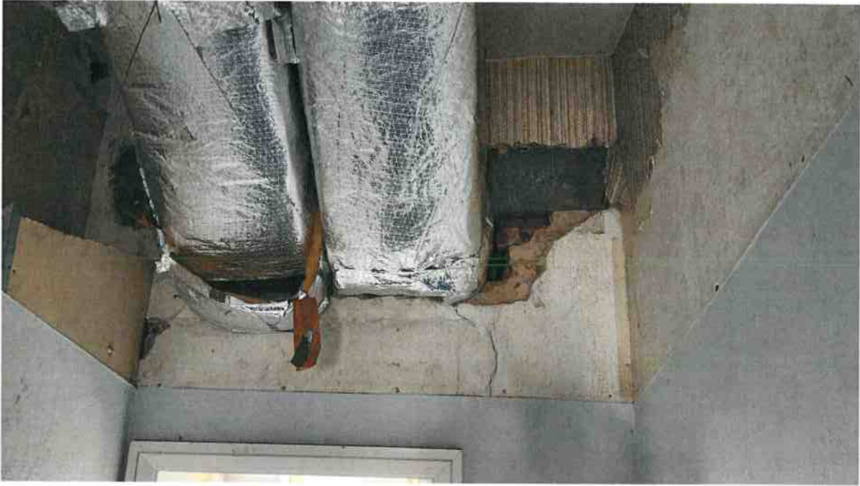
Significant structural damage caused due to inappropriate construction from the past.
