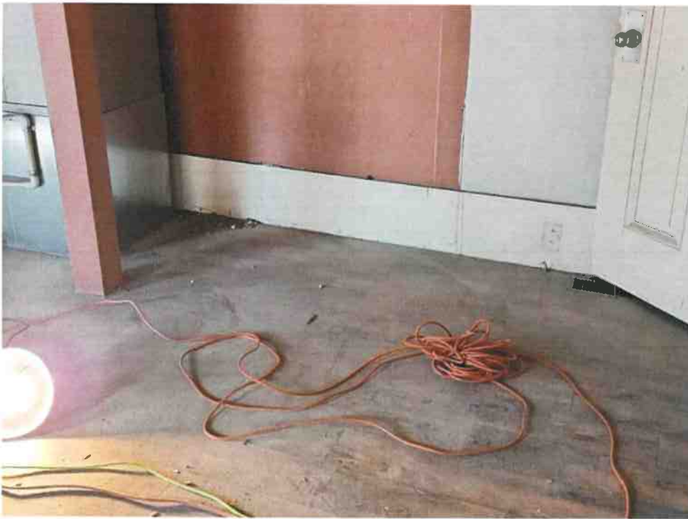
Sunk floor (picture does not capture the issue very well but the issue is evident when looking at it in person)
