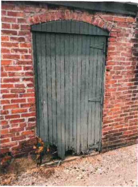
Water damaged door in Fountain Alley on Donkey Barn
