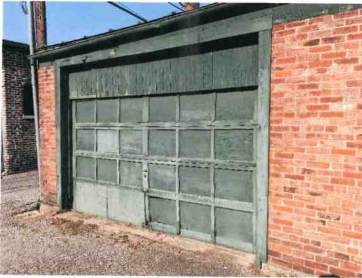
Garage door in poor shape with rotted wood frame
