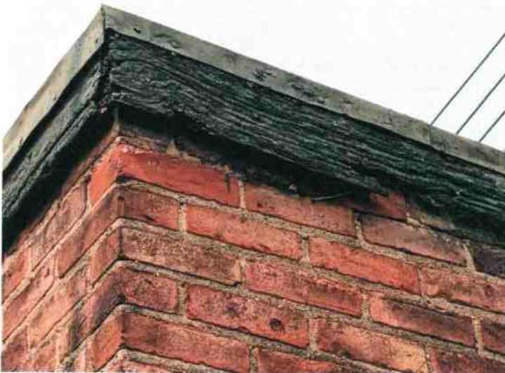
Rotted fascia boards on both buildings
