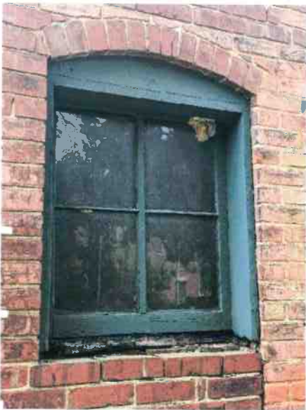
Window on North side of garage needs repair
