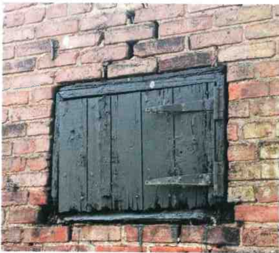
Rotted frame and window covering on North side of garage
