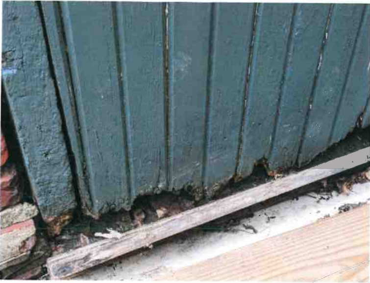
Water damaged door North side of Donkey barn
