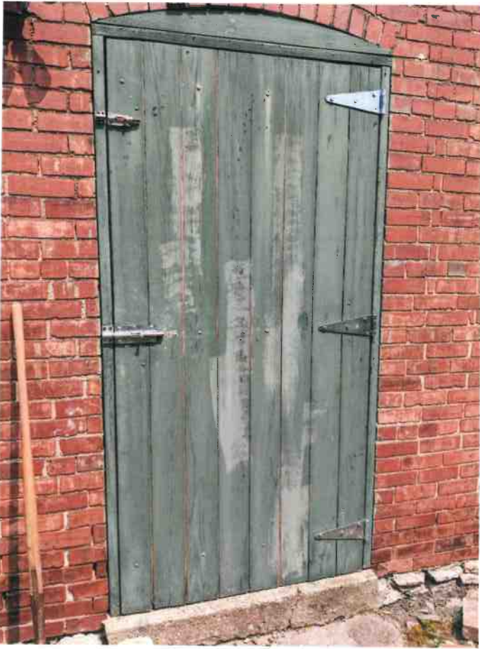
Door on West side of garage is difficult to bolt shut
