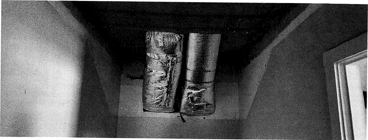
Lot of damage caused due to the duct work (Example of inappropriate alterations)
