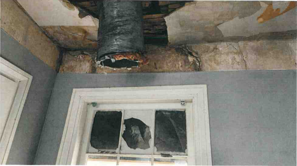
More examples of cracks in the walls and plaster.
